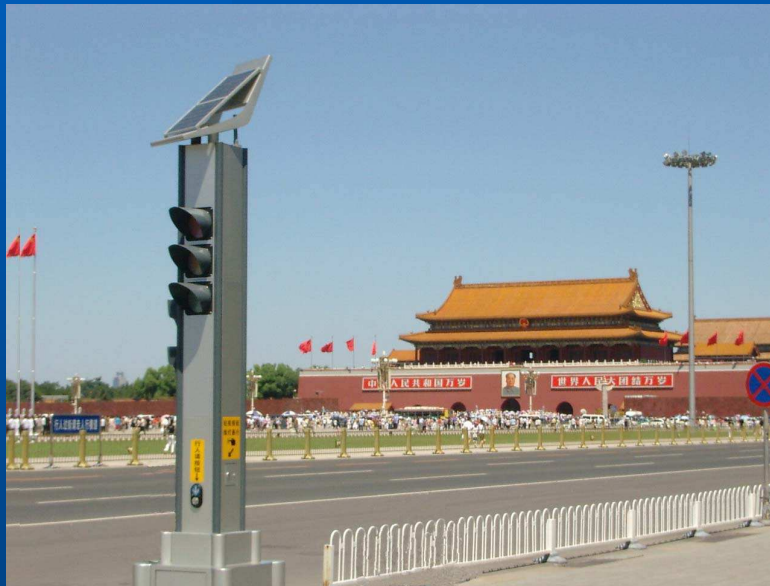
Solar Traffic Signals
