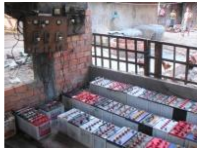
Battery charging in Cambodia
