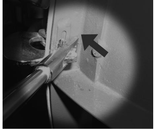
Wrong lock position
